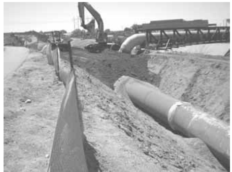
Large diameter pipeline installation parallel to Albuquerque Metropolitan Arroyo Flood Control Authority's North Diversion Channel.
