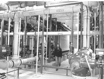
Below - inside the arsenic microfiltration plant. At right - repairing a steel water line.
