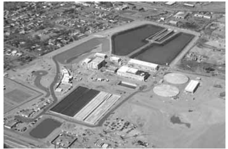
Above is an aerial photo of the drinking water treatment plant at 75% completion.
